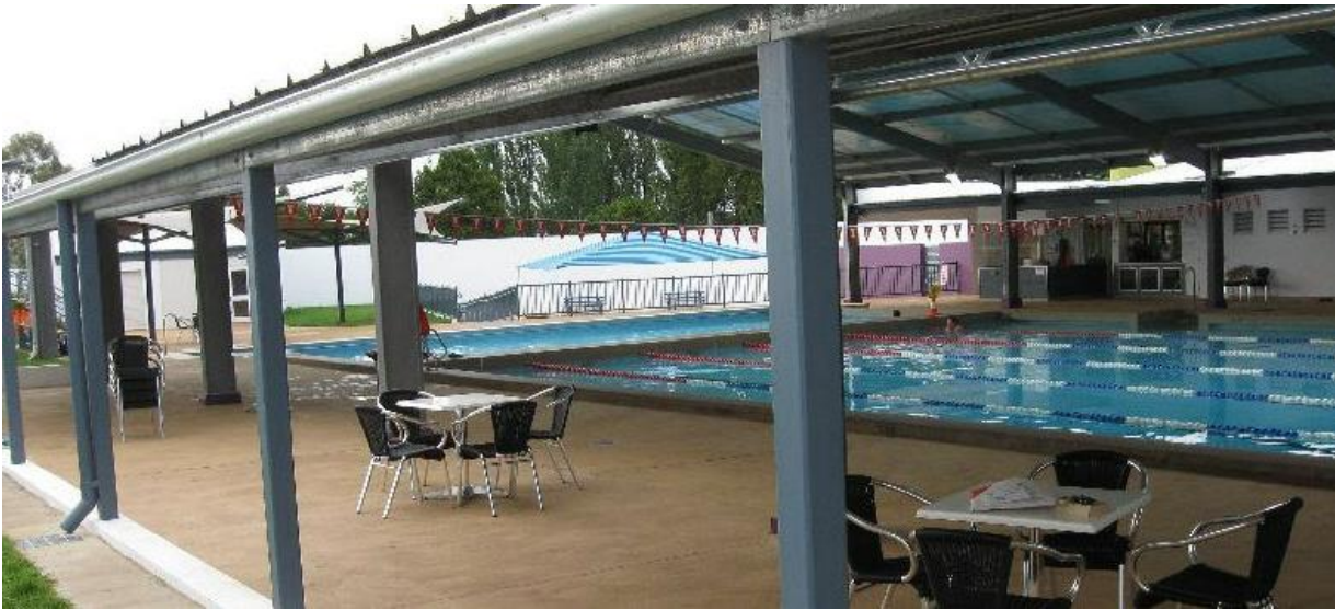
Figure 7: The existing skillion roof was built in the 1994 upgrades and is proposed to stay.
